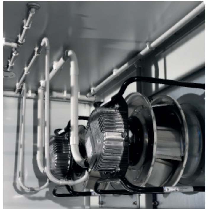
Fig 22. Power and signal cable conduits
